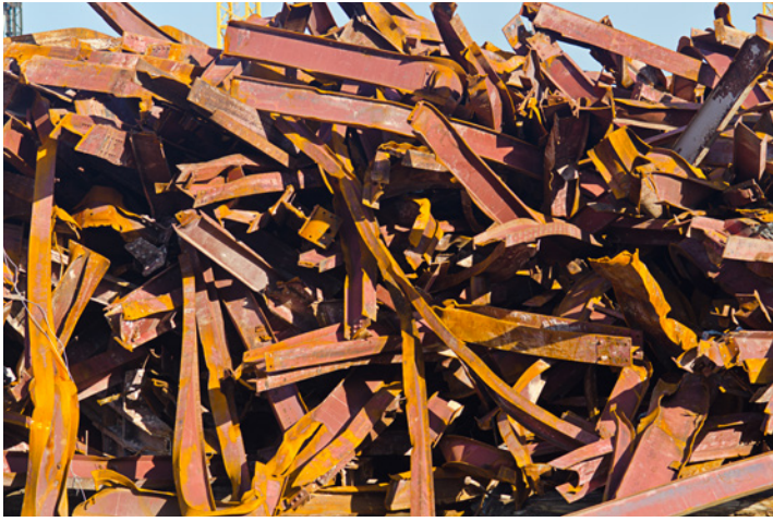
Debris from the demolition of the Grand Palace Hotel/Claiborne Towers building, New Orleans.
